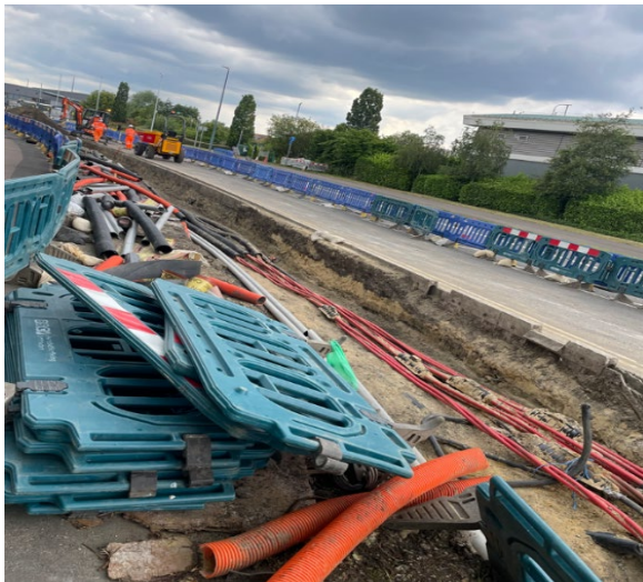
Exposed utility cables from north east corner
