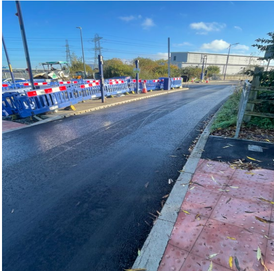
Photo of the outbound approach of the Kent Fastway which has recently be resurfaced.
