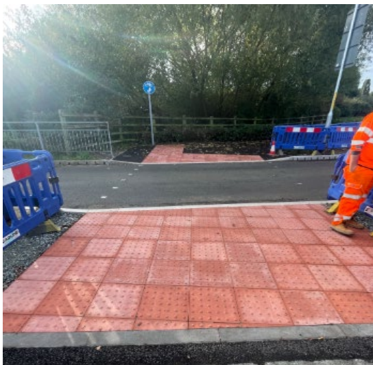
New tactile paving that has been laid across Kent Fastway pedestrian crossing point.
