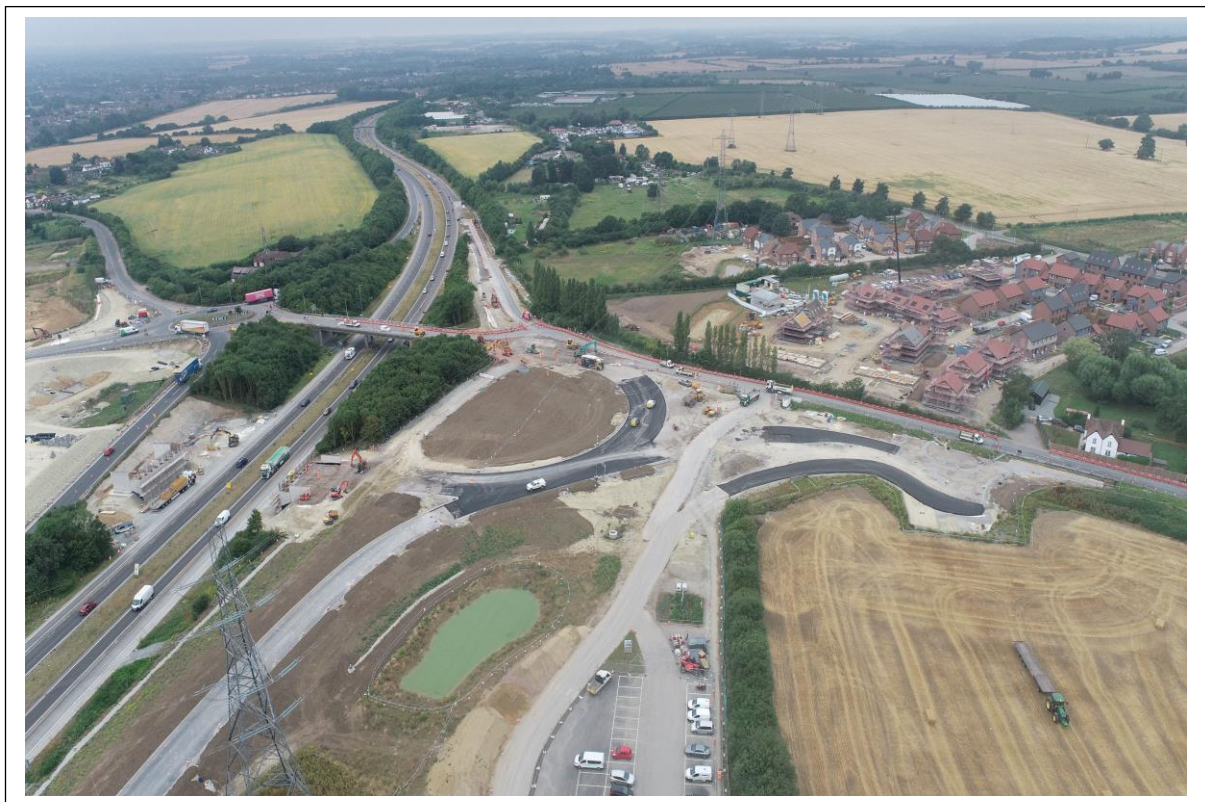
Aerial view of works on the bridge walls, northbound slip roads and Grovehurst Road north roundabout.
