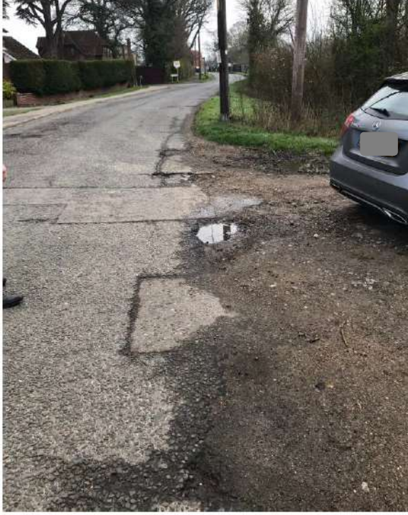
Pothole at construction entrance
